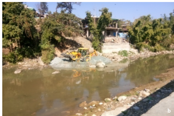
Image 3. a—Habitat degradation by mining activities near Jullang village | b—Earth work by JCB machine for construction of wall at Police colony, Itanagar, Arunachal Pradesh. © Lakpa Tamang.
