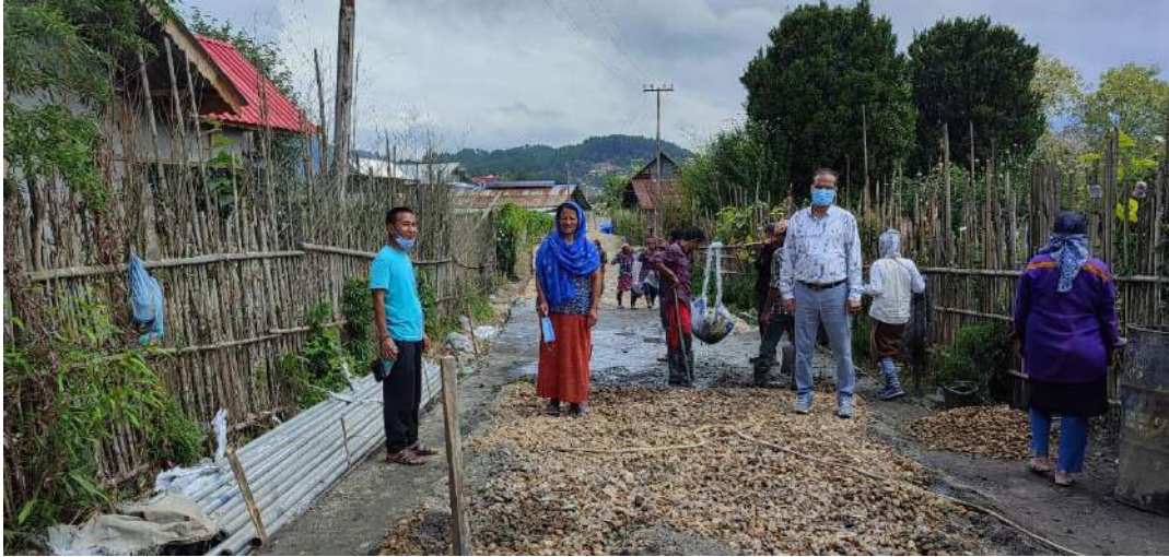
Construction of CC Road at Hija Village under Ziro-I CD Block, Lower Subansiri District (Source: Block Office, Ziro-I CD block, Dated 18/05/2019)
