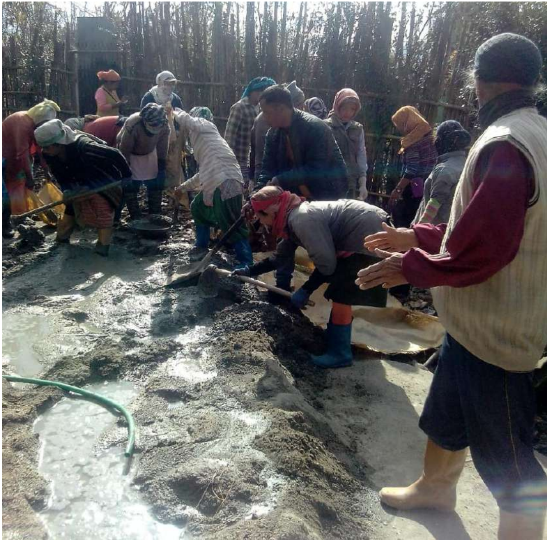
MGNREGA Workers preparing Cement for Construction of CC Road at Lempia Ayo Myolyi, Gram Panchayat, Ziro-I CD Block, Lower Subansiri District.
