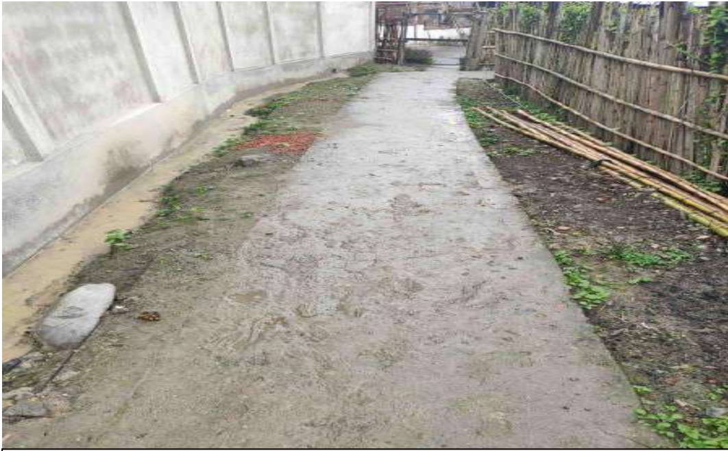
CC Footpath constructed under MGNREGAat Diirii Hapa, Sululya West Gram Panchayat, Ziro-I CD Block, Lower Subansiri District. (Source: Field Work at Sululya Village, Dated 13/05/2019)
