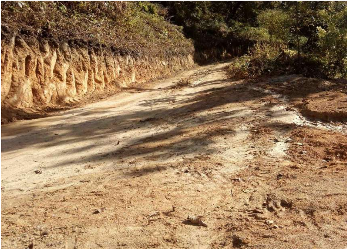
Link Road Constructed connecting Pre village to Hara Village under MGNREGA at Jara Gram Panchayat, Ziro-II CD Block, Lower Subansiri District. Source: Field Work at Jara GP, Dated 18/07/2019
