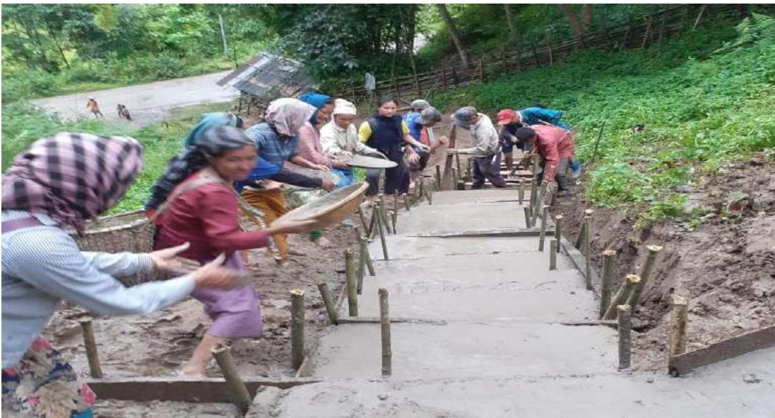
Constructed of CC footpath under MGNREGA at Jara Gram Panchayat, Ziro-II CD Block, Lower Subansiri District. Source: Block Office, Ziro-II CD Block, Dated 18/07/2019
