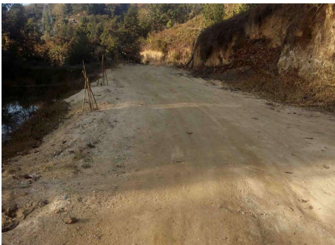
Link Road Constructed connecting Peil Village and Nyuth Village under MGNREGA at Joram Gram Panchayat, Ziro-II CD Block, Lower Subansiri District.
