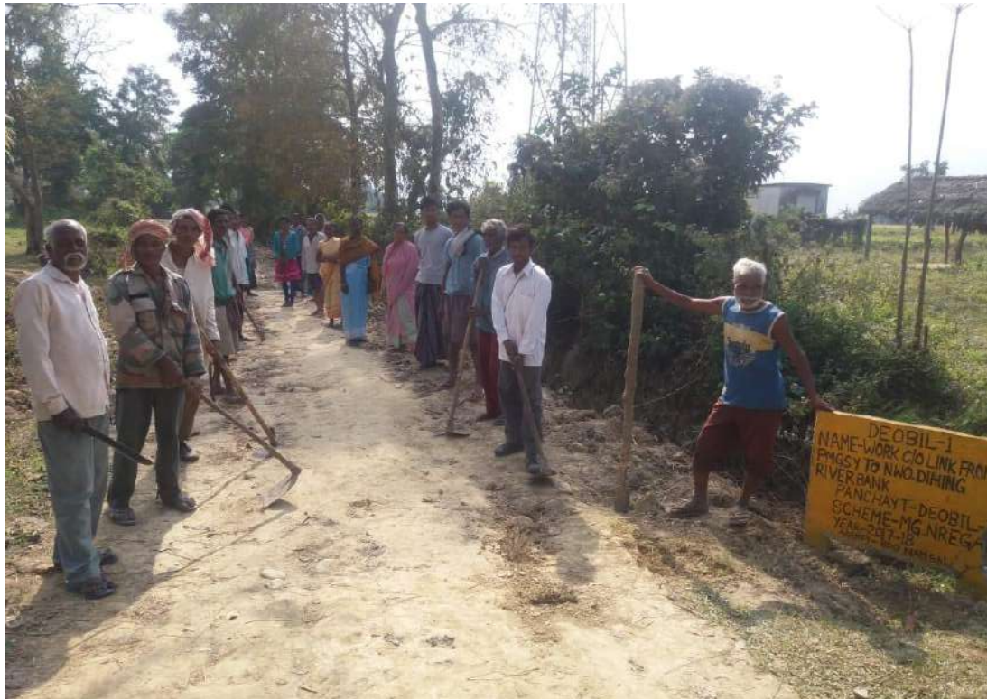
Link Road Constructed from PMGSY Road to Nwo-Dihng River Bank under MGNREGA at Deobel-I Gram Panchayat, Namsai CD Block, Namsai District.
