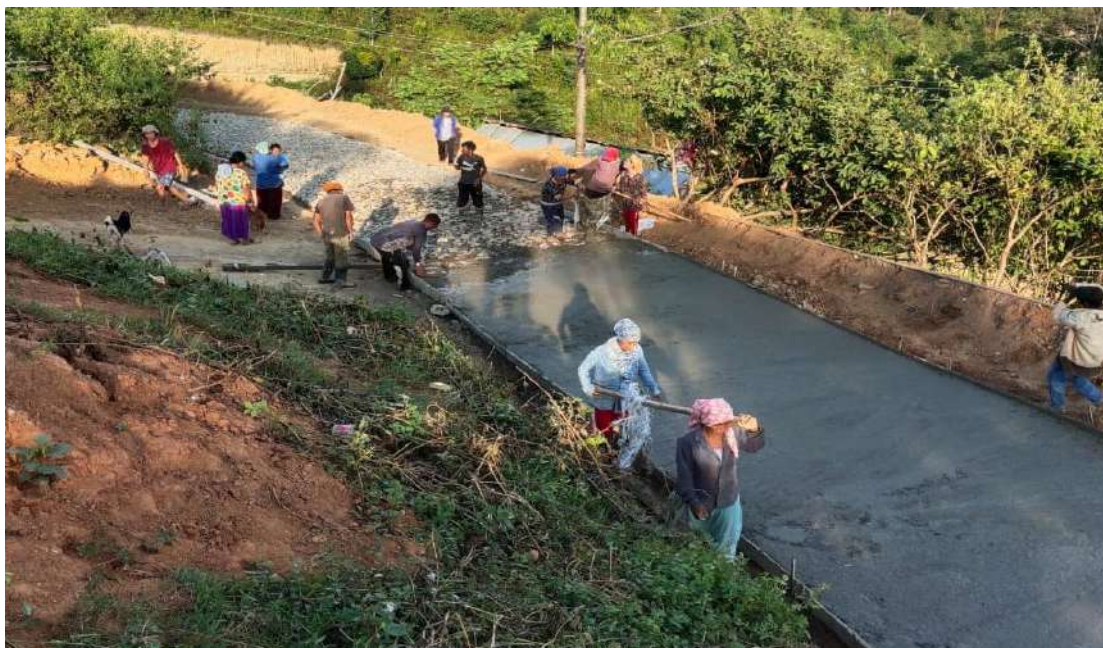
Construction of CC Footpath under MGNREGA at Toon Village, Joram Gram Panchayat, Ziro-II CD Block, Lower Subansiri District.
